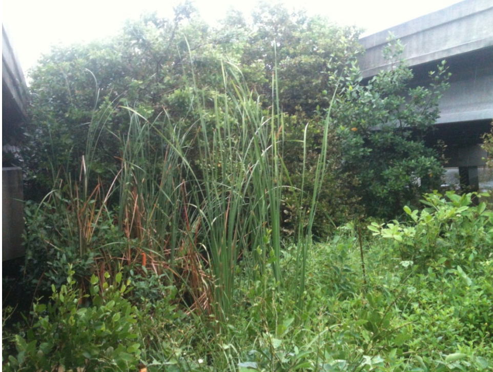
Photo 9. South bank of the North Fork of the New River between the mainline Bridge for the northbound lanes and the entrance ramp
